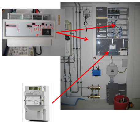
Figure 3: Installation of Prosumer Household Measurement and Control Equipment (above: GridSense box, below: L+G 350 SmartMeter)
